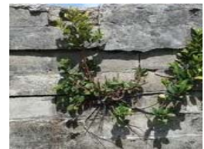
Do remove plants and roots that are growing into a wall. You might have to poison the plant in order to ensure the plant in order to ensure it does not regrow
