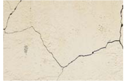
Hard concrete plaster often cracks when covering softer more pliable masonry
