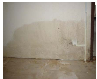
Rising Damp caused by the removal of a suspended wooden floor and replacement with a concrete slab
