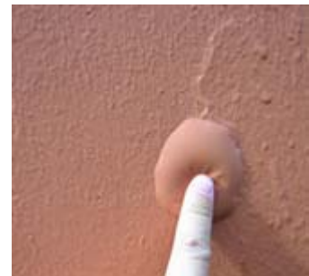
Use of paint that does not breathe caused blistering as it traps the moisture in the walls
