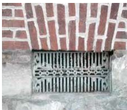
Do keep your ventilations grills clear to allow air to circulate below your wooden floor
