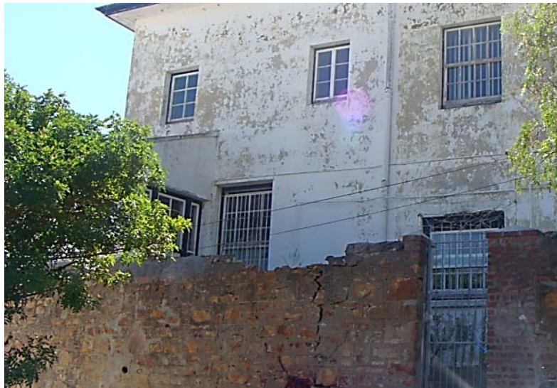
Lack of simple maintenance to a building such as this will end up causing significant damage to original features and materials and incur much larger expenditure (Simon's Town)
